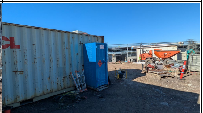
Dangerous goods stored in robust banded dedicated stores.
