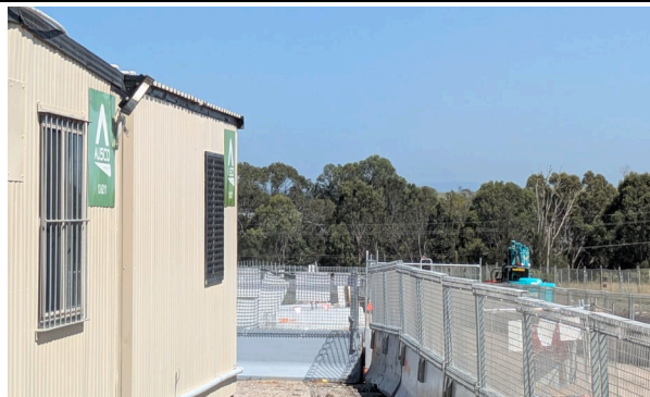
Site compound luminaires aimed down.
