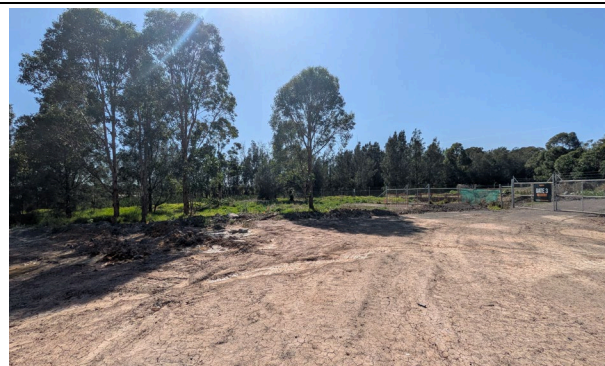
Eastern boundary and no-go zone flagging was missing but was installed the same day.
