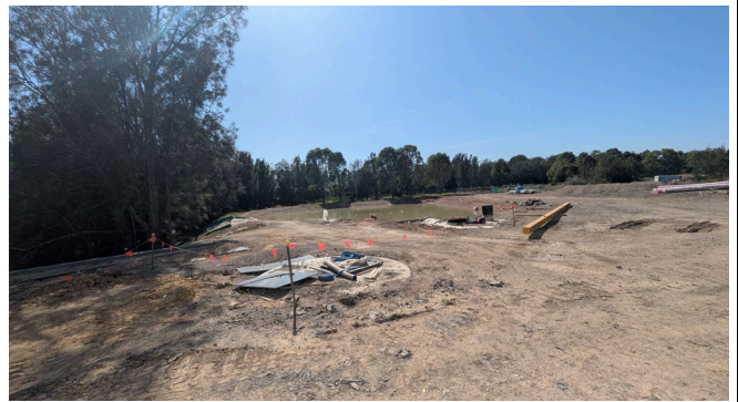
SE Sediment basin well constructed, and stormwater pit headwall works in the foreground.
