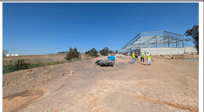
Earth berm along eastern third of southern boundary required well shaped and stable.
