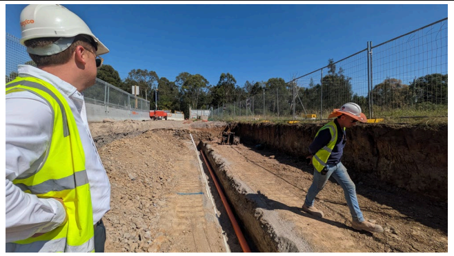
Northern half of site access road to Adams Road installation of stormwater system and services - work self-contained.
