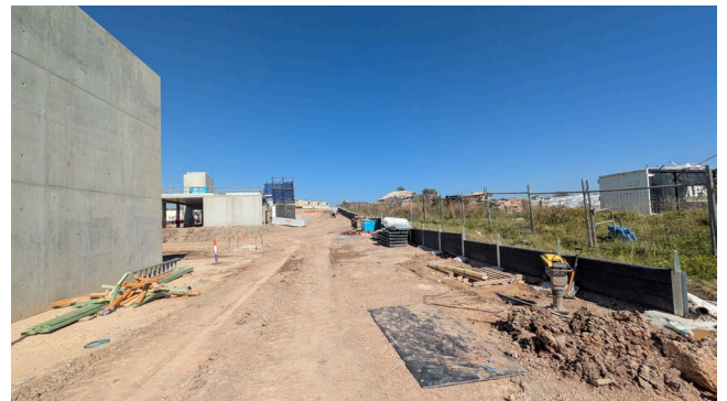
Northern boundary - View west along push walls of retaining wall and stormwater system installation works.
