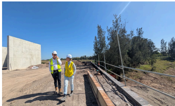
NE and East retaining wall and stormwater works ensure site is self-contained.
