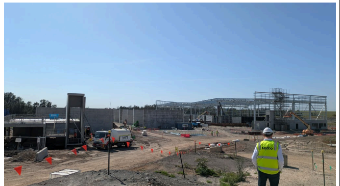
General view of construction site to the southeast – site is well planned, controlled and organised.
